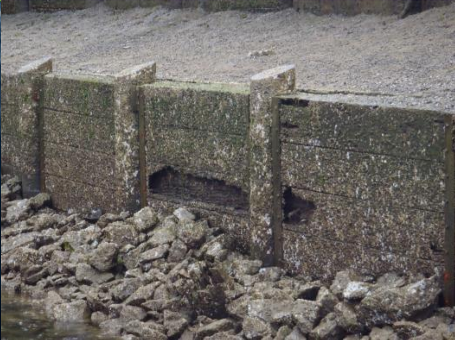
Current Lagging Degradation
